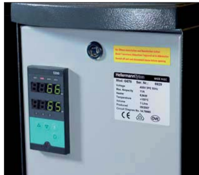
Professional type plate on a heating unit.
