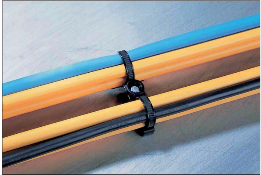
Parallel fixation of two cables.
