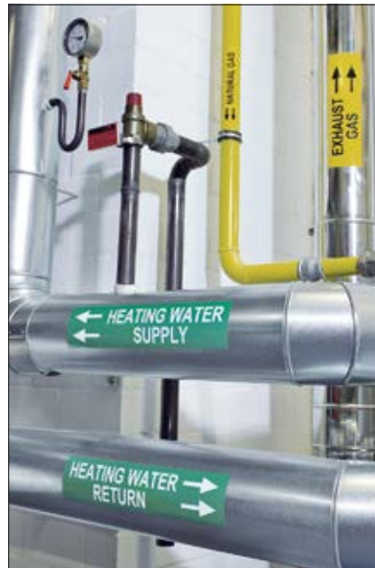
Large and highly visible pipe marking.
