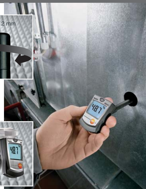
Monitoring air humidity in an air conditioning duct
